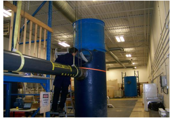
Standpipe on inlet side of the stormwater testing lab
